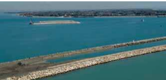
3. Malamocco inlet. The outer breakwater and the construction of the lock for large ships
